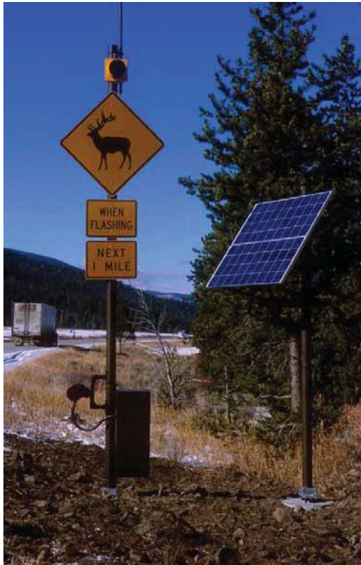
Figure 38. Photo. Animal detection system along Highway 191 in Yellowstone National Park, MT (copyright: Marcel Huijser, WTI).
