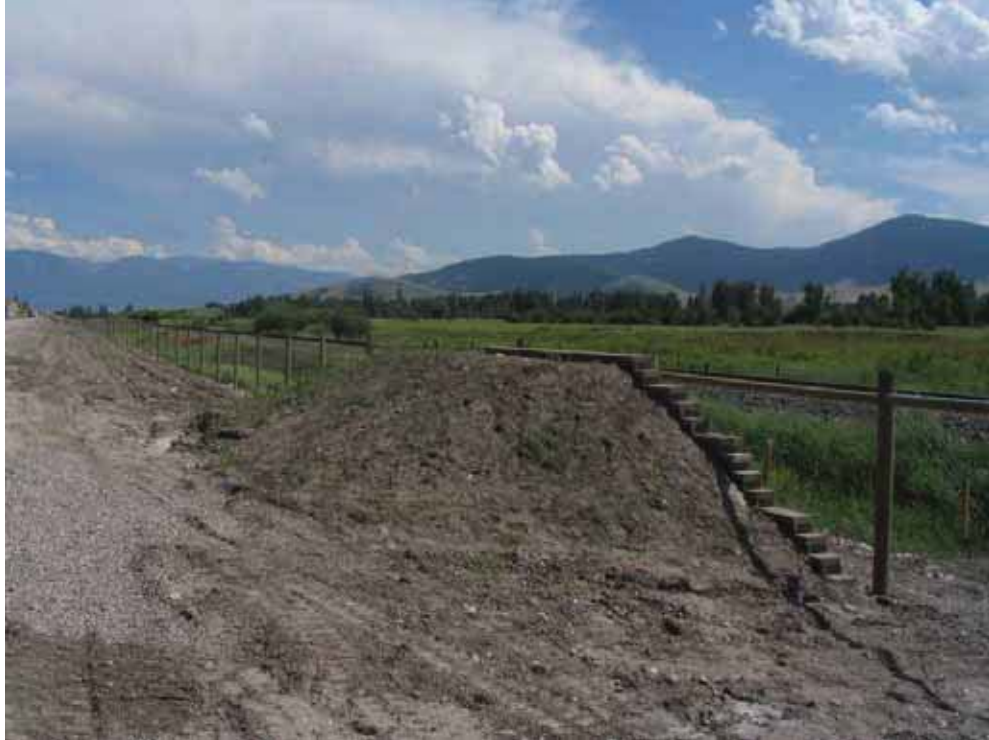
Figure 48. Photo. Jump-out or escape ramp along U.S. Highway 93 on the Flathead Indian Reservation, MT (copyright: Marcel Huijser, WTI).
