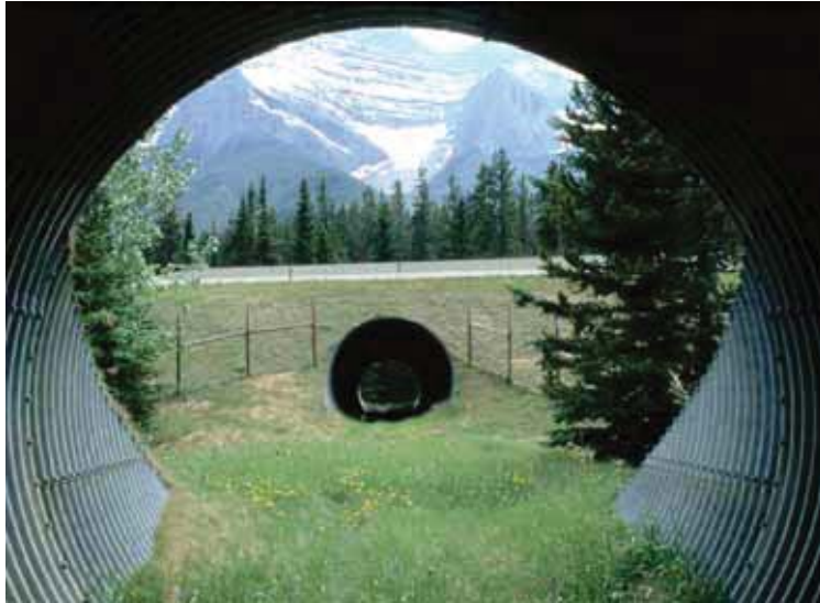
Figure ES15. Photo. Large culvert with vegetative cover and fencing on Highway 1 in Canada (copyright: Tony Clevenger).
